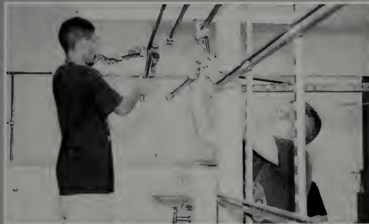
PJ Perry and Carl Santino learn how to correctly install a gas line in Plumbing Shop.
